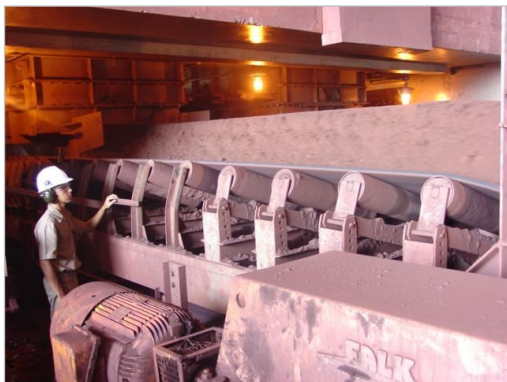
Fig. 3. One of the feeders under the bin.
